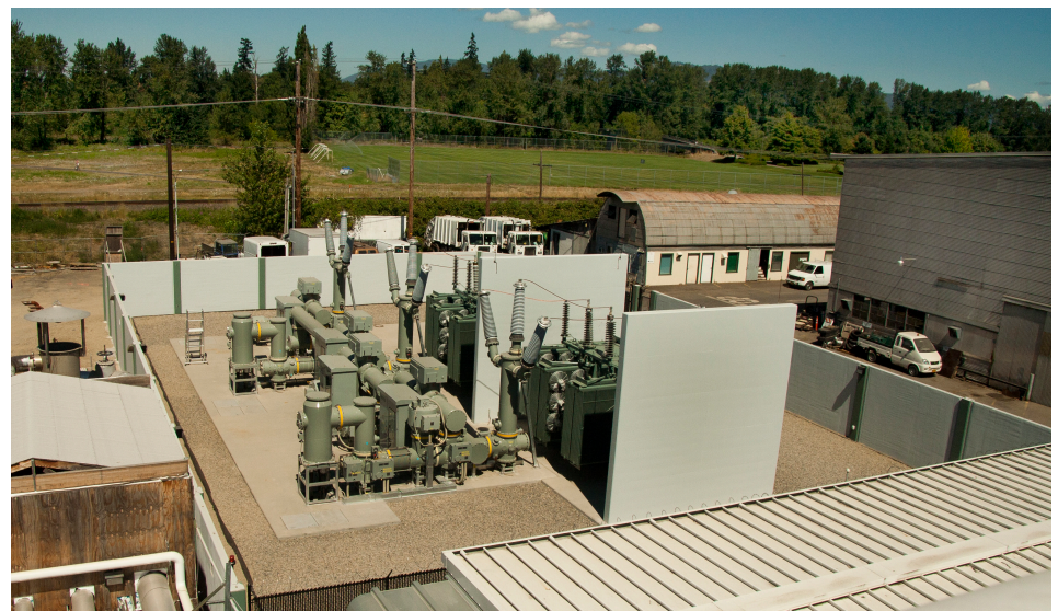
The dual-redundant electrical substation incorporates the latest technology to serve campus.
