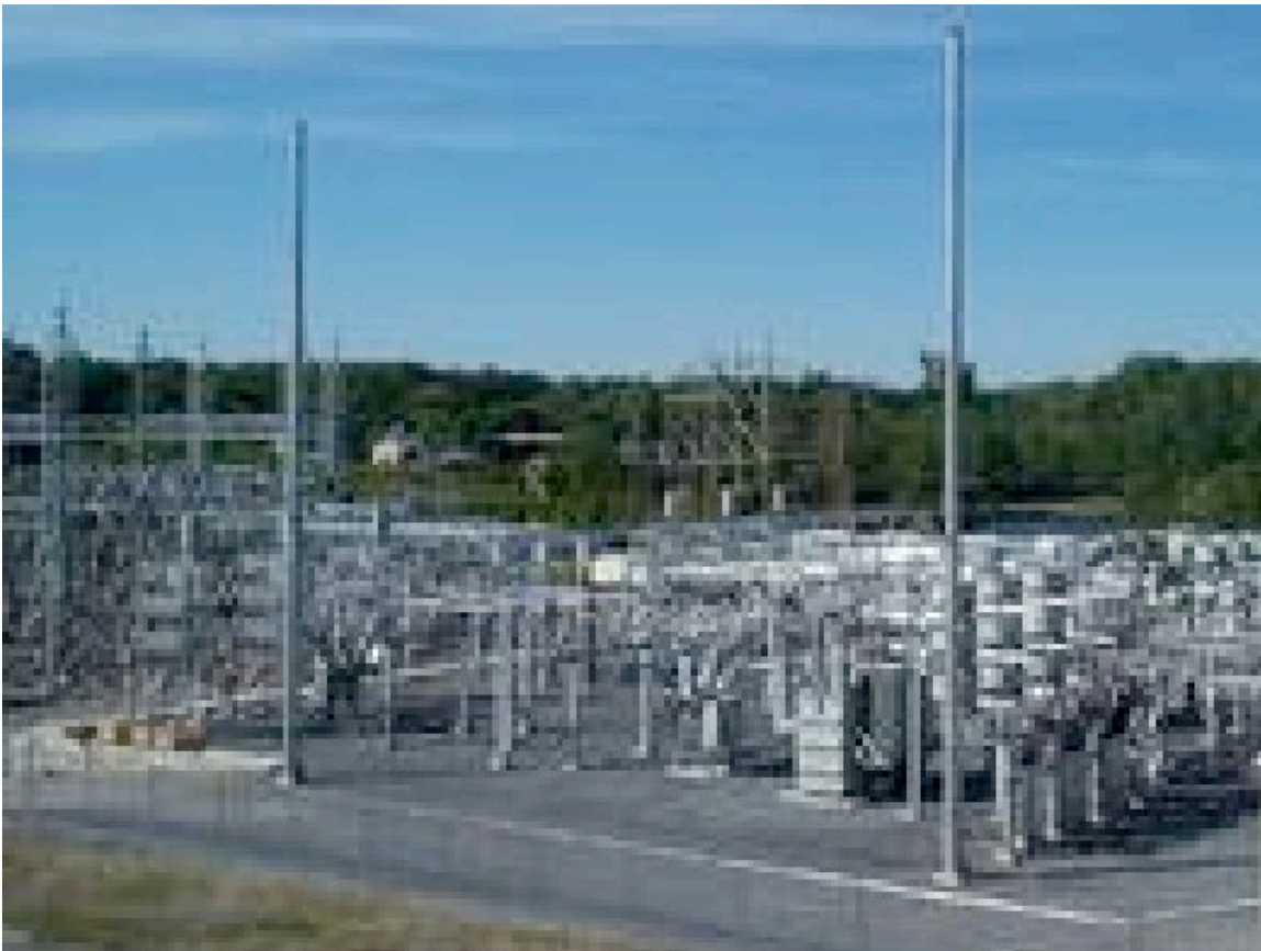
Figure 7. In 2001, Vermont Electric Power Co. installed a Mitsubishi Electric Power Products STATCOM system at its Essex substation to combat voltage instability and power quality problems (Appendix 2).
