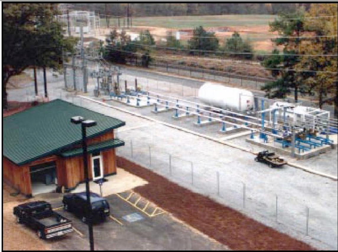
Figure 9. High temperature Superconducting cable installation, switchyard, and control room from Southwire.
